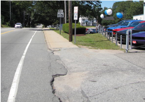
RIPTA stop on Toll Road at Bald Hill Road/Route 2 in, Warwick, RI has a driveway in the landing area
